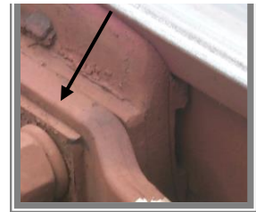
No gap between point & stock rail
