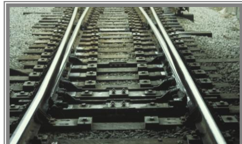
Gap at both switch points will de-rail a train
