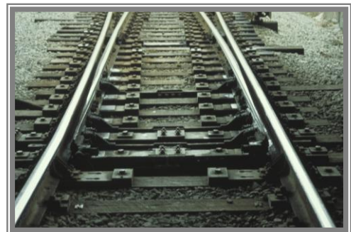
Gap at both switch points will de-rail a train
